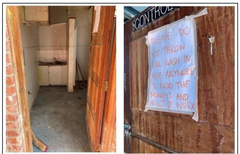
Figure 12. Problematic waste room that has been cleared and is no longer in use at Waterfall barracks.
